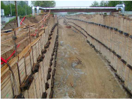
Fig. 1 Open pit for the cut-and-cover tunnels between the Střížkov and Prosek stations
